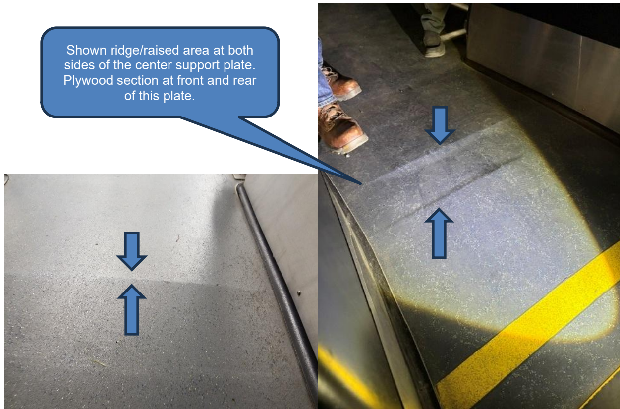
FIGURE 2: SHOWN VIEW OF FLOORING RIDGED/RAISED AT AFFECTED AREA
