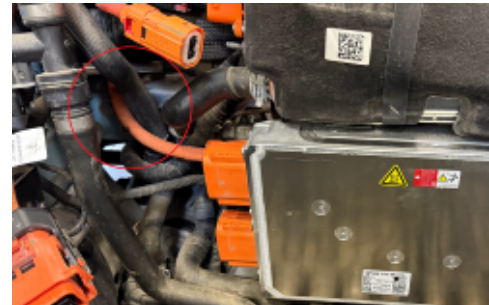
Live high-voltage line
