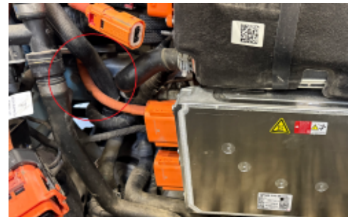
Live high-voltage line
