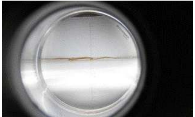
Figure 4. Paintwork crack evaluation using a magnifying glass.
