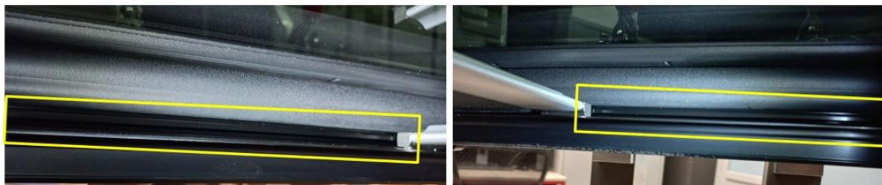
Figure 2 Contamination of roof / guides for sunblind slide shoes
