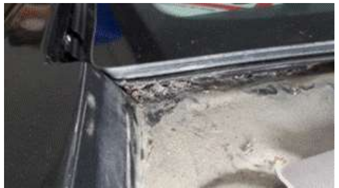
Figure 4. Water drain channel blocked by dirt.
