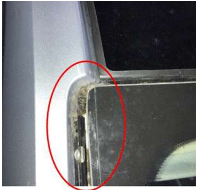
Figure 7. Dirt in exposed channel.
