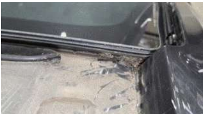
Figure 3. Water drain channel blocked by dirt.
