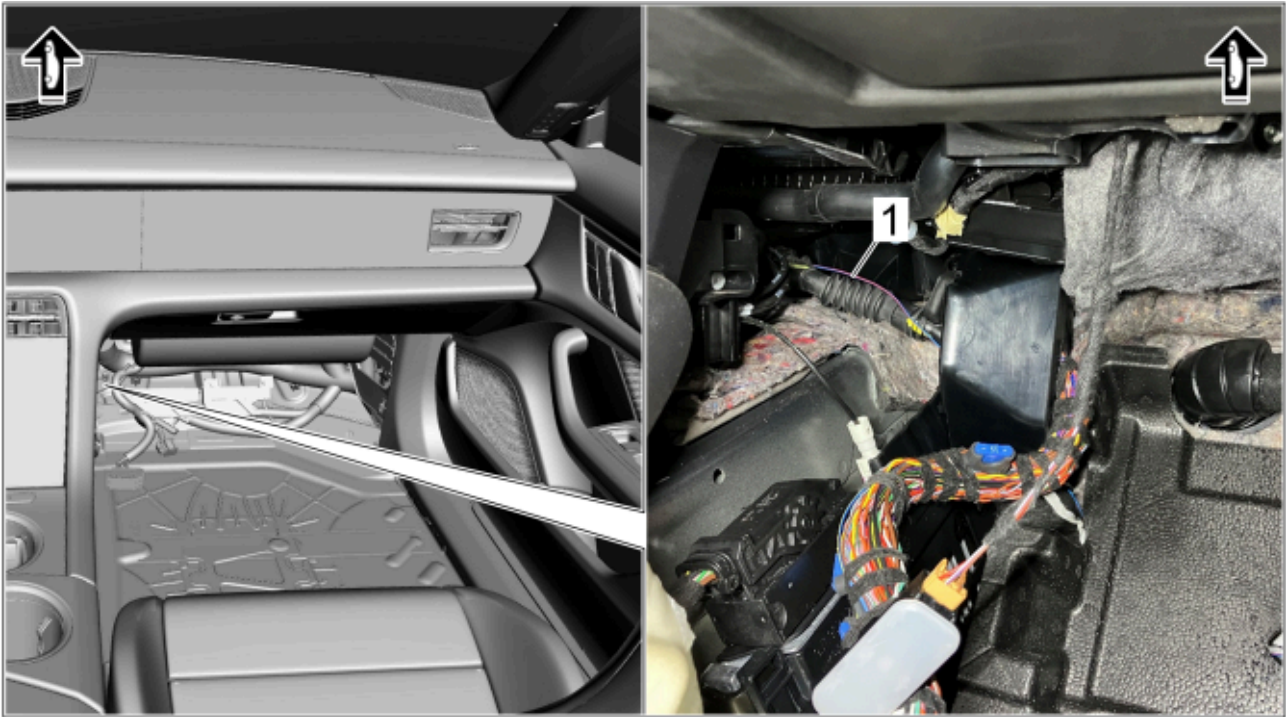
Electric wire harness under dashboard
