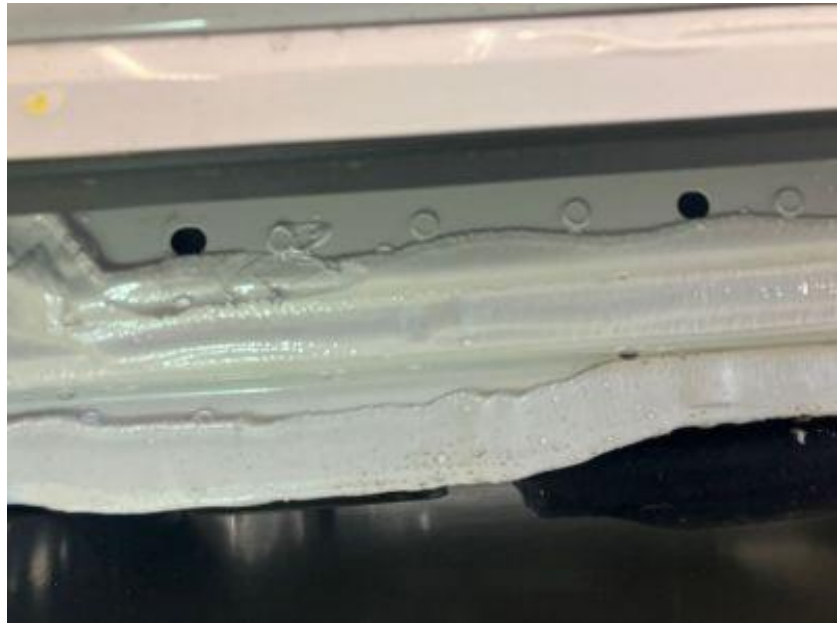
Figure 3. PVC joint seal too high.
