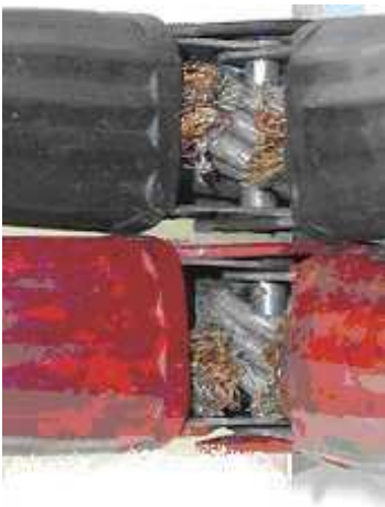
Figure 1. Copper bridge in clamps cracked.
