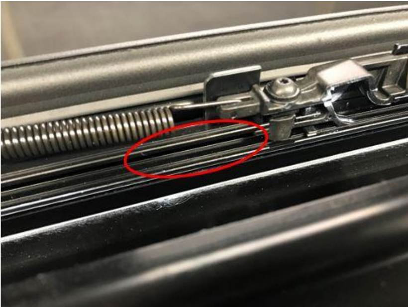
Figure 25. The section of the rail guide to be cleaned is circled in red.
