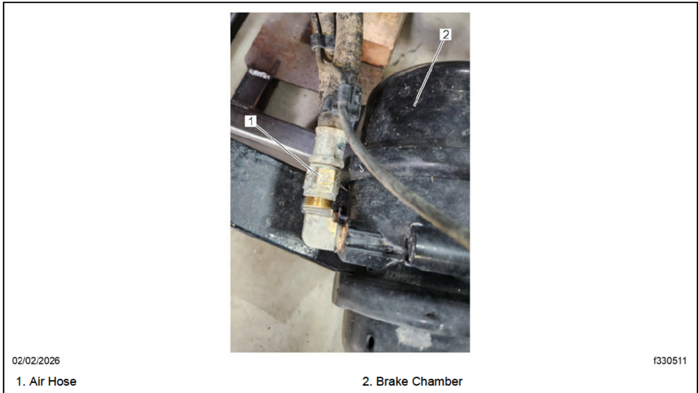
Fig. 2, Air Hoses Connected to the Brake Chambers
