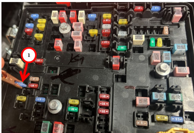
Fig. 1 F08 MOD Cluster Fuse Location
