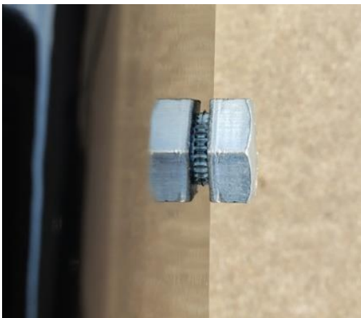
Poorly Seated Bolt
