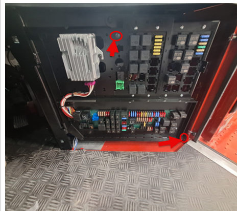
figure 2, open electrical board
