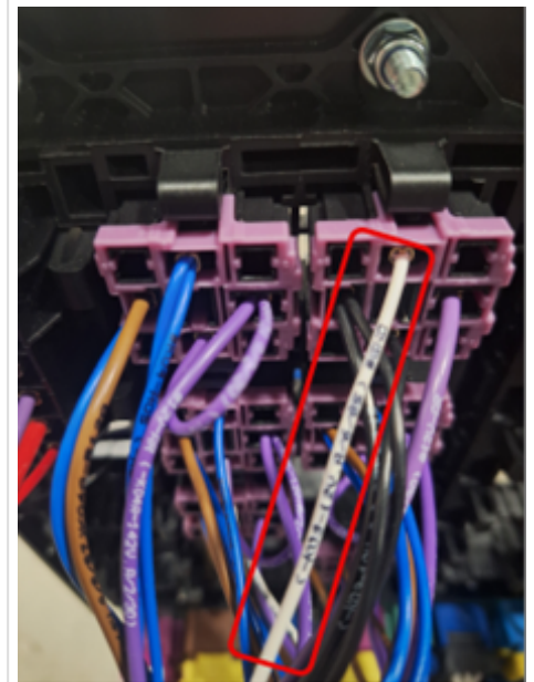
figure 4, check labels on wiring
