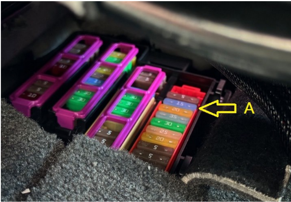
Figure 2. Fuse control panel
