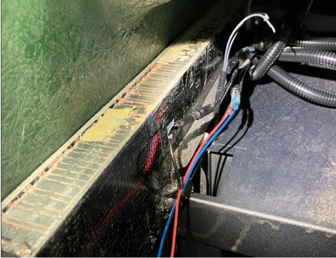
Photo of New Wires Under the Step
