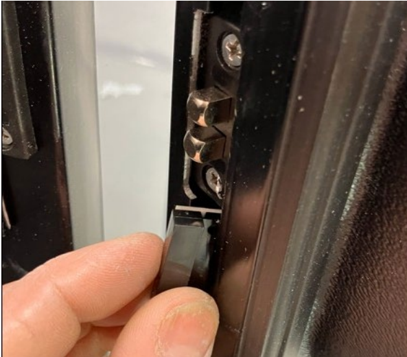
Step 14- Placement Of Sensor On The Door
