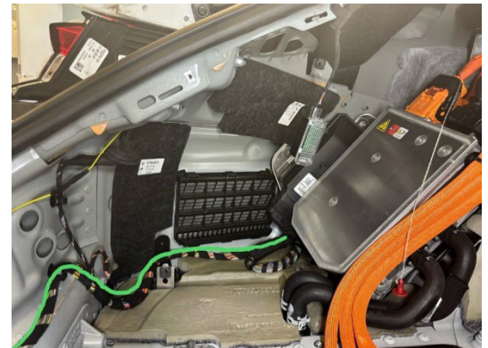
Figure 15. Driver-side Trunk Area Routing
