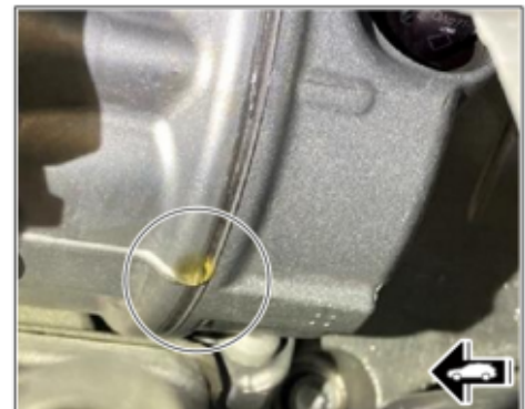
Drop formation on air-conditioning compressor
