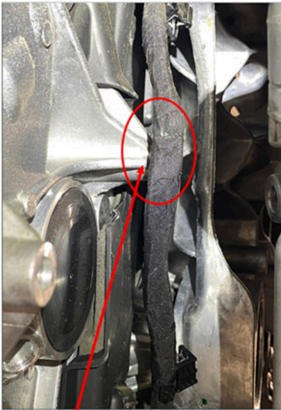
Wiring harness chafed with body near rear e-ATS
