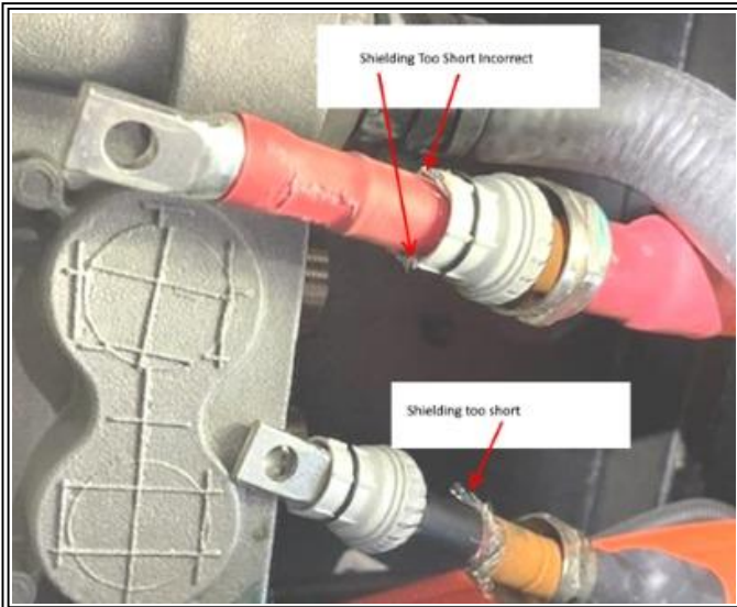
Figure 5:DC Cable shielding too short
