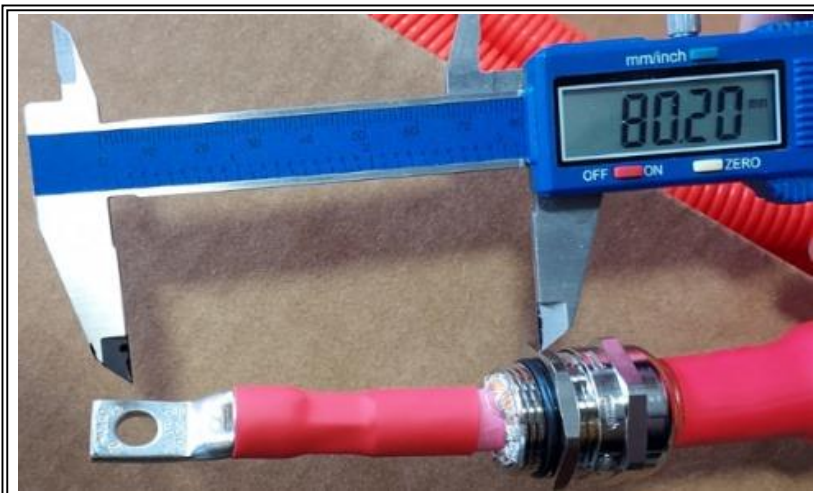
Figure 11:DC Cable measurement out of spec 80 mm do not use.
