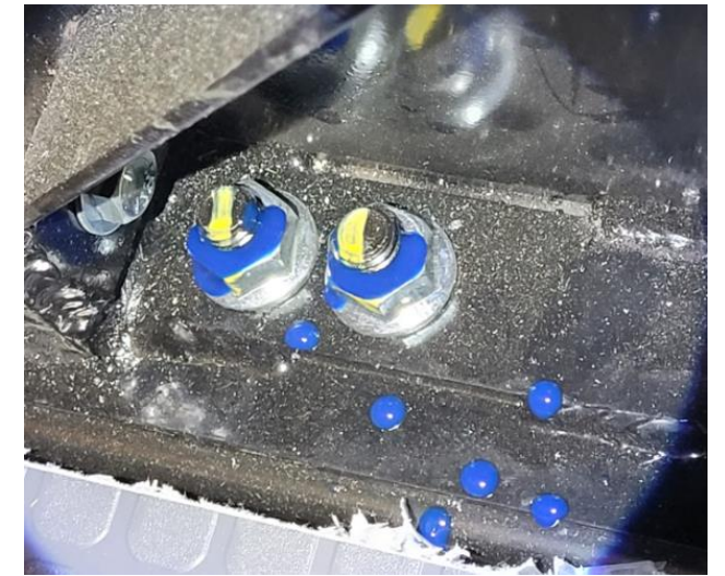
Figure 14: Correct Loctite coverage is on top of the nut at least halfway around.
