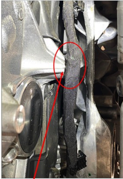
Wiring harness chafed with body near rear e-ATS
