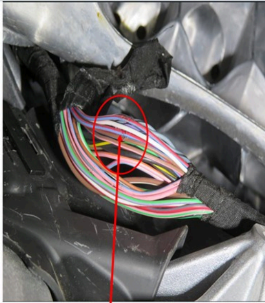
Wiring harness cut near rear e-ATS
