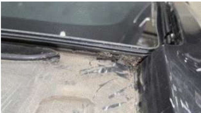
Figure 3. Water drain channel blocked by dirt.
