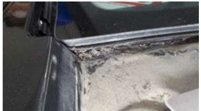
Figure 4. Water drain channel blocked by dirt.
