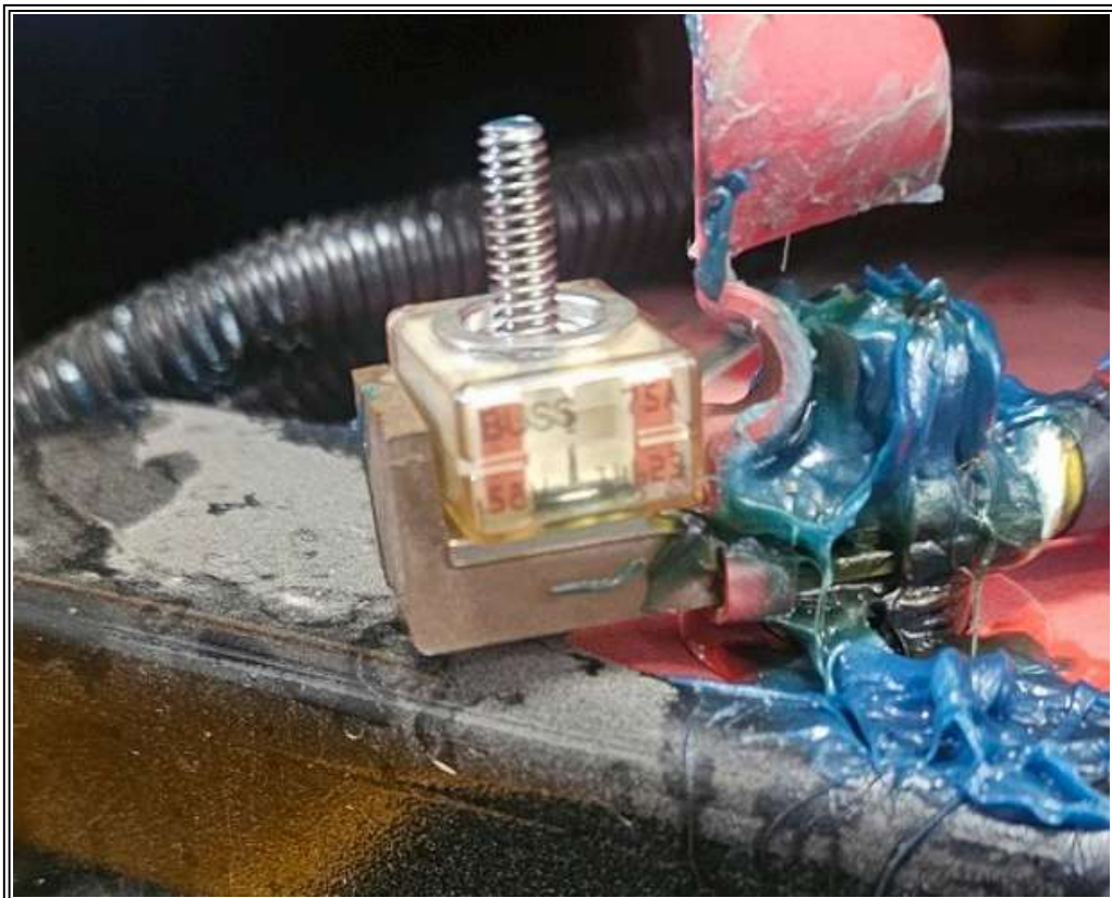
Figure 1: Incorrect 75A Fuse
