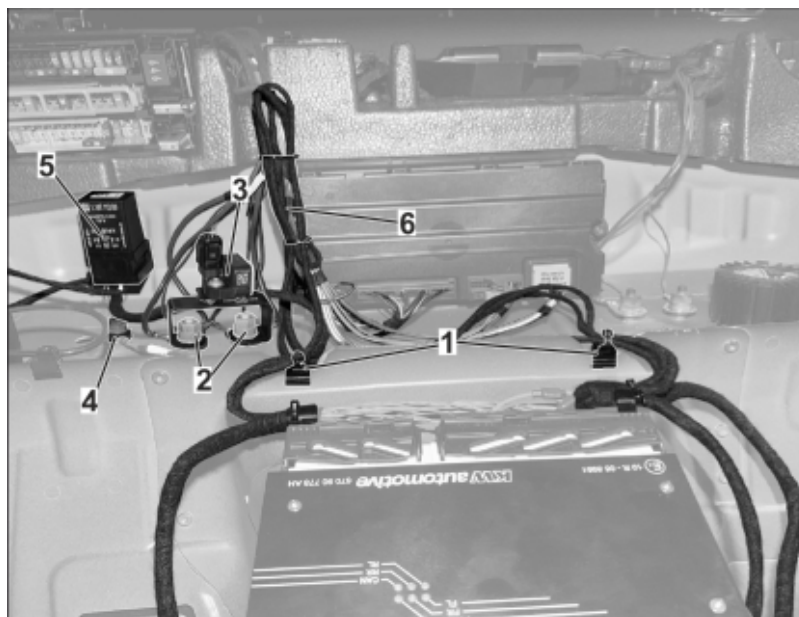
Cable routing in interior area of control unit
