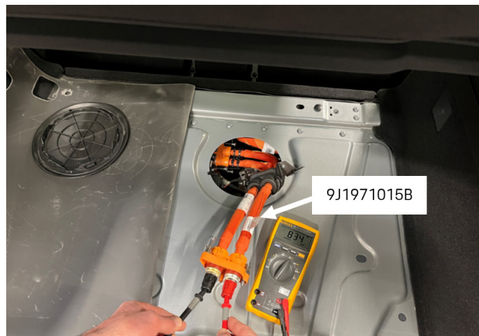
Figure 4 - Measuring Capacitance on Rear PE
