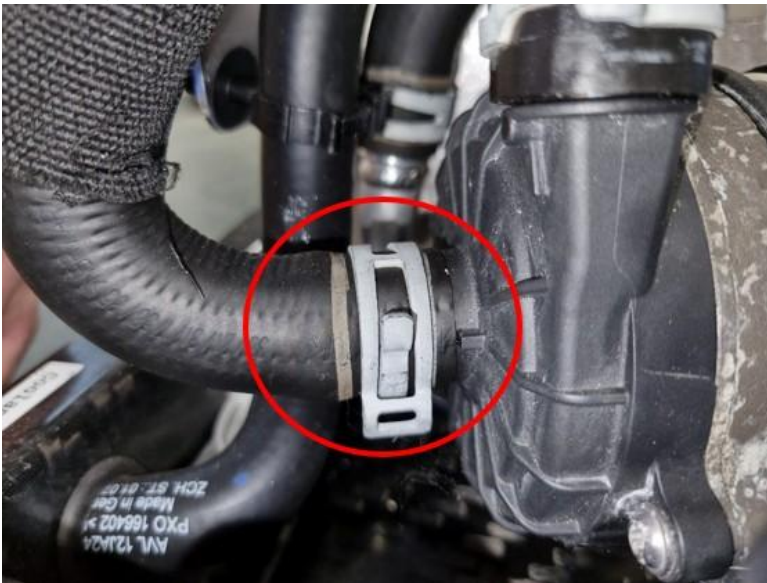
Hose to pump inlet interface
