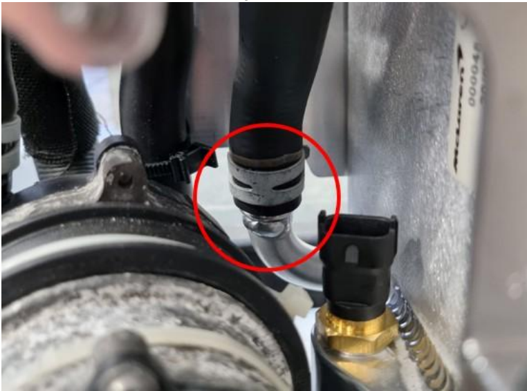
Hose to heat exchanger interface
