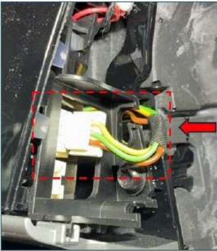
Figure 1. Incorrect wire routing.
