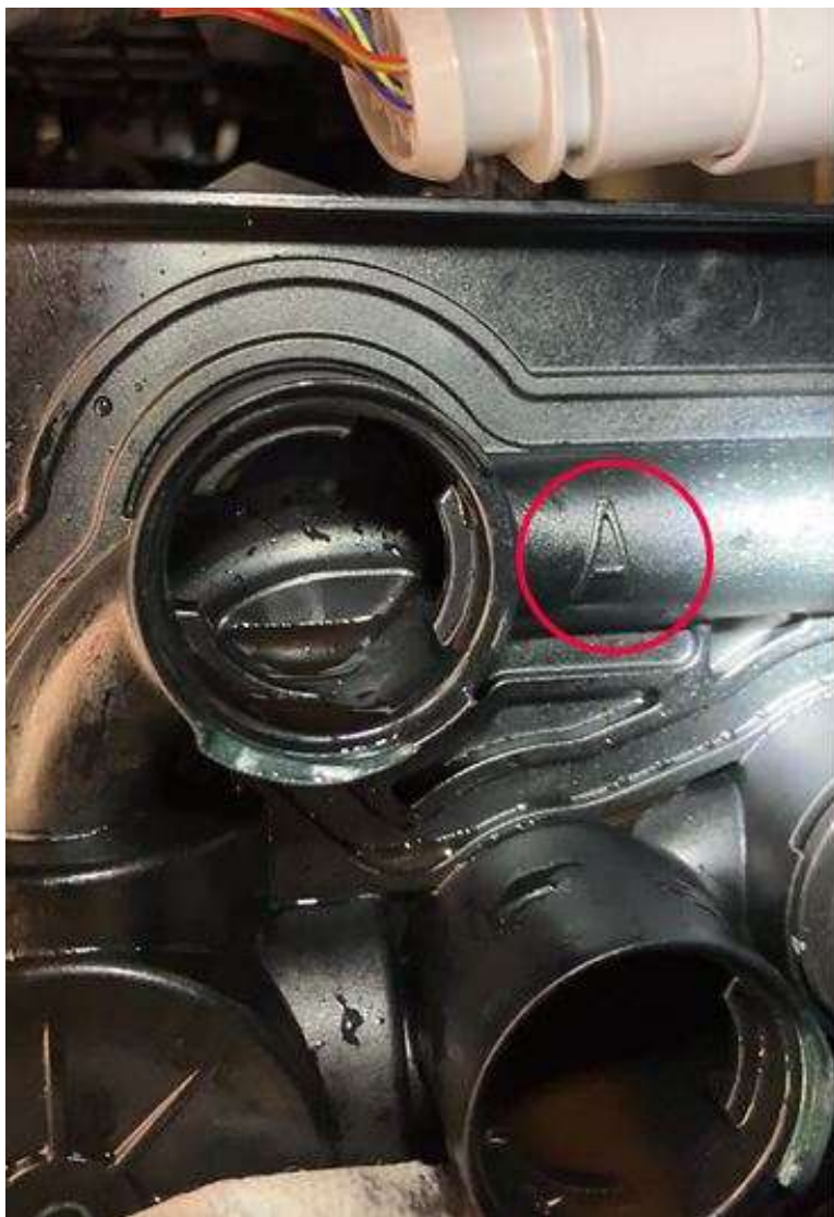
Figure 1. The label on the hose connection on the coolant distributor.
