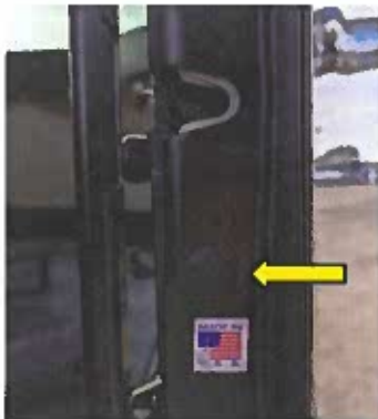
Figure 1 – Solid plastic plug, needs to be replaced
