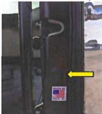
Figure 1 – Solid plastic plug, needs to be replaced
