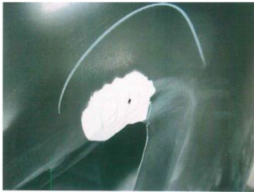
Grind top side at least 1 inch by 2 inches ( depending on crack size )
