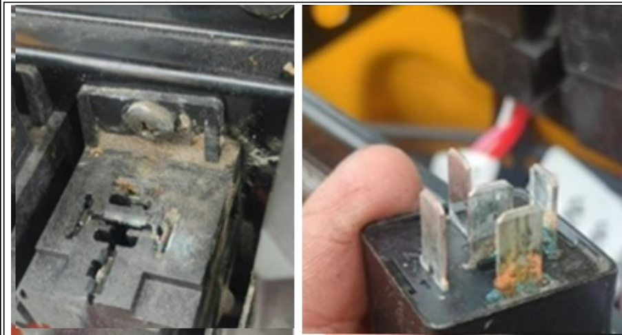
Figure 3: Corrsion Relay Socket and Relay Terminals
