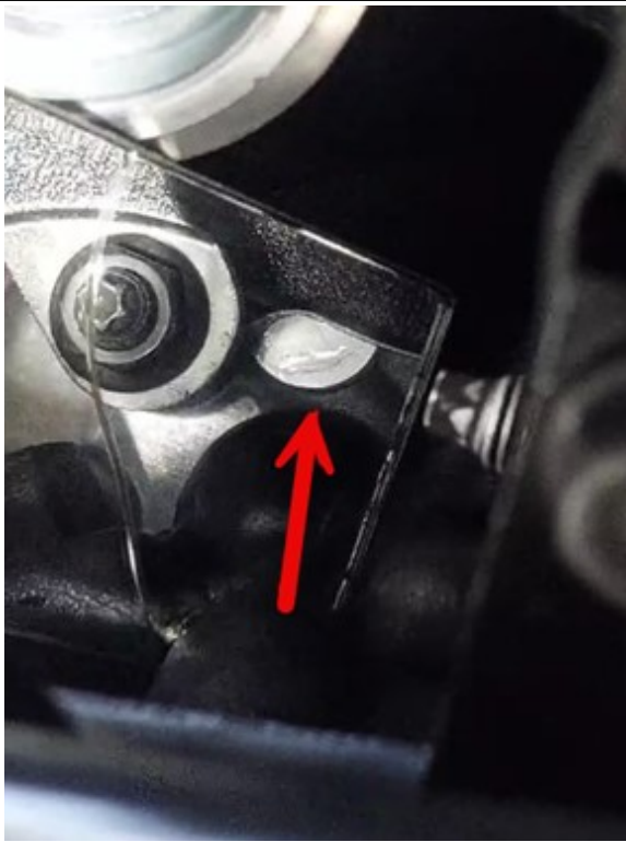
Figure 2 - Gear Housing Boss Leak
