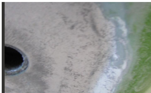
Pitting Found After Sanding Example (Fig. 1)
