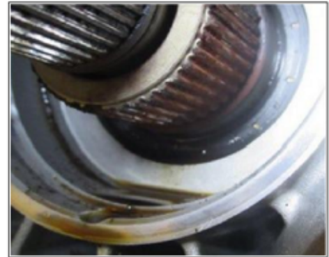
Oil leakage on output-shaft sealing ring
