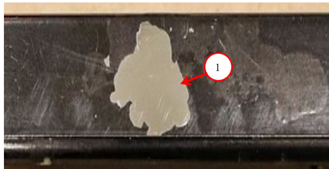
Fig. 2 Paint Peeling Example
