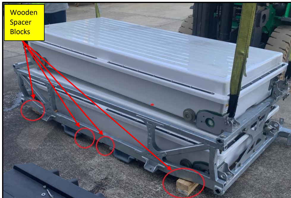
Figure 22: ESS Battery Packs Wooden Block Under the Assembly Location Reference.
