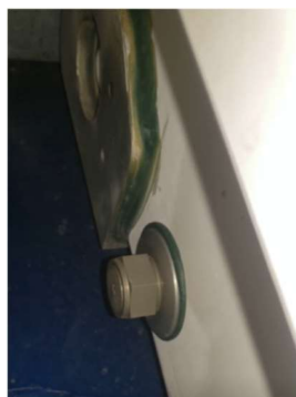
Figure 3A: ESS Drain
