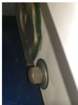
Figure 3A: ESS Drain
