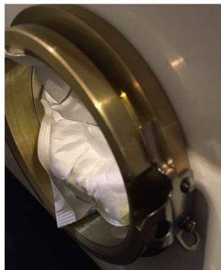
Figure 12: Desiccant Bags to be Removed
