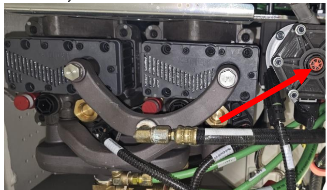
Dryer system with oil separator
