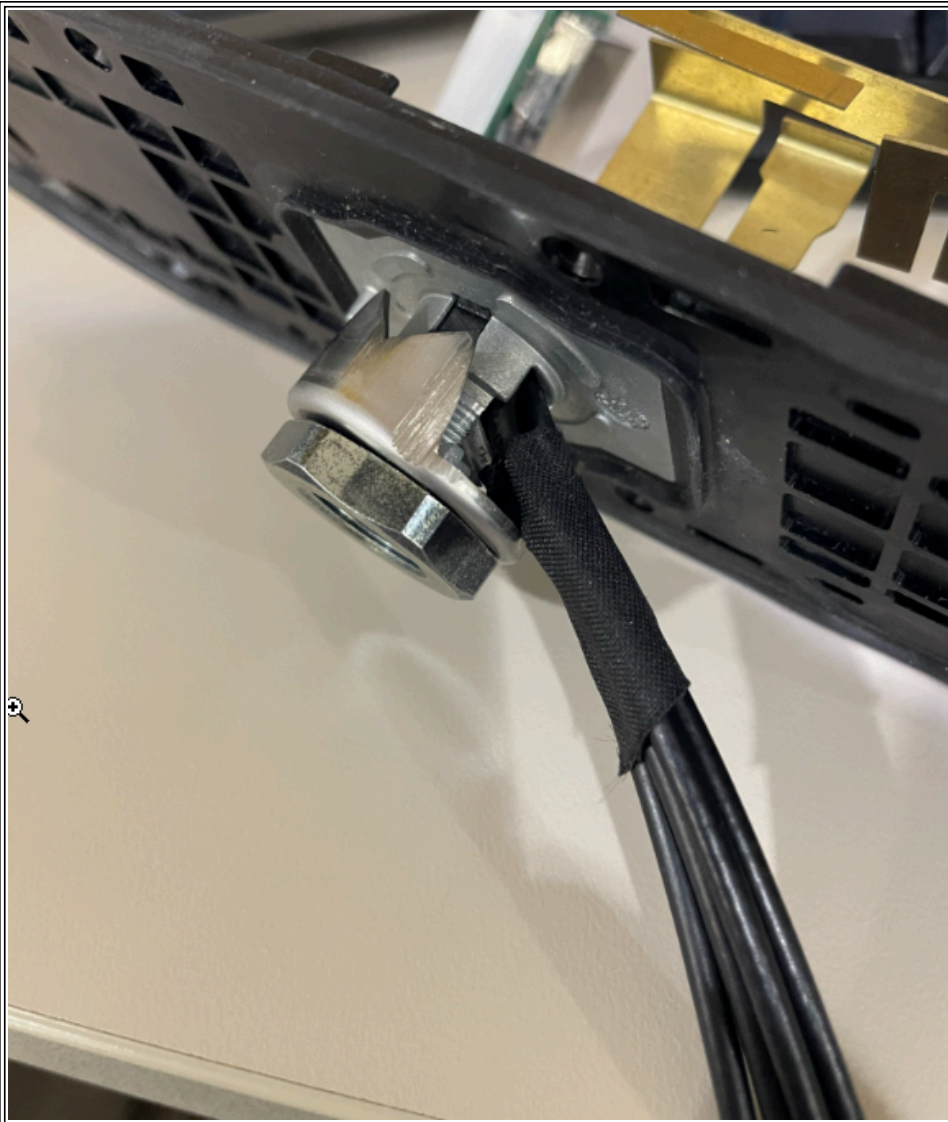
Figure 3: Cables Protected with Friction Tape
