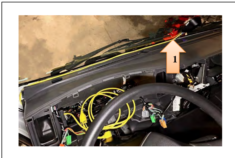
Figure 23 Current Cable Routing (painted yellow for reference) 1. Tape Location
