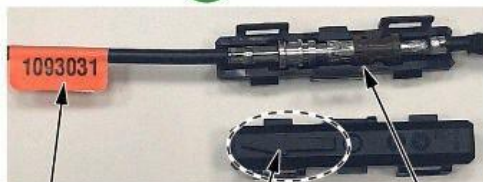
RED FLAG LABEL Arrow facing toward tag. Fully seated in splice box.
