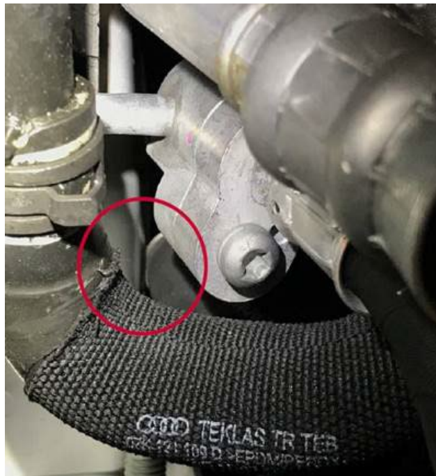
Figure 2. Refrigerant line in contact with longitudinal member.
