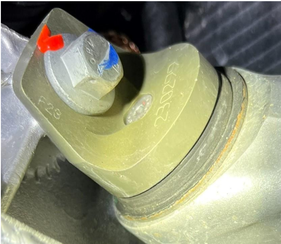
(Example 1 - Bush outer metal dirt accumulation.)
