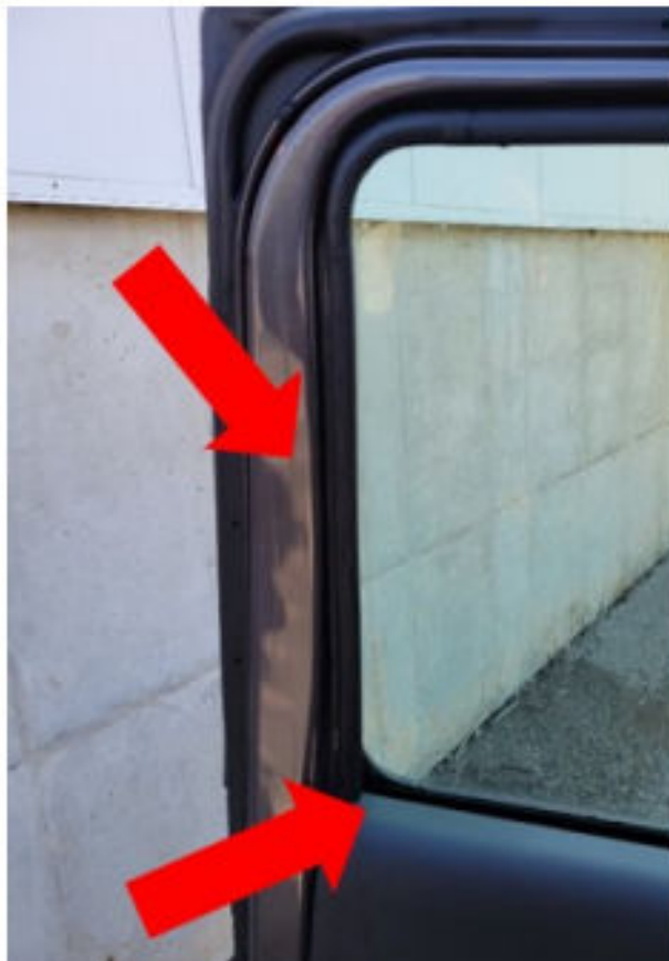
Fig. 1 Water Drip Area Down The Inside Door And Panel
