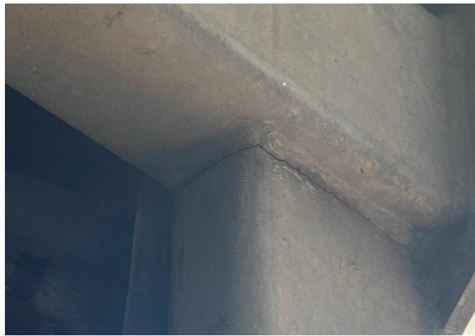
Example crack at upper corner of rear frame
