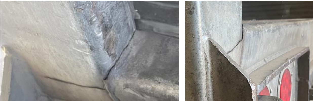
Example cracks in lower corners of rear frame
