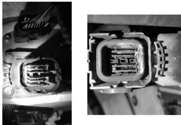
Figure 9 Battery Pack Connectors - Failed w/Heavy Soot)
