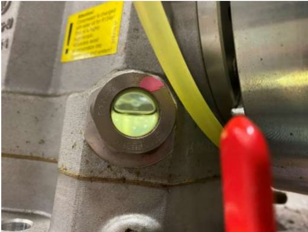
Figure 4: The oil pan of the HVAC compressor is illuminated through the opposite sight glass
