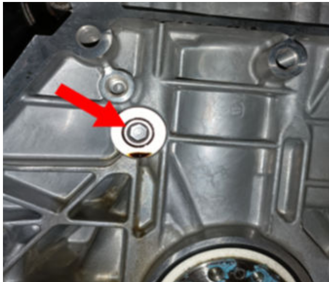
Fig. 1 Oil Valley Cap Leaking
