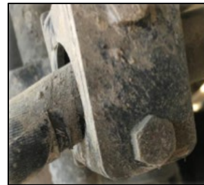
Figure 2. INCORRECT Use of Tube Clamps for Hoses
